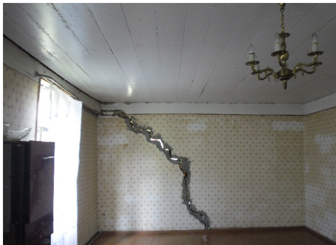
Figure 9. Village Dgvari, house damaged by landslide.
