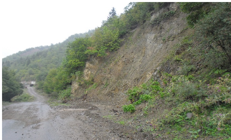
Figure 18. Rockfall (Chobiskhevi road).
