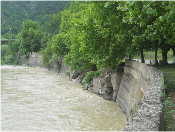
Figure 7. Riv. Mtkvari right bank erosion.
