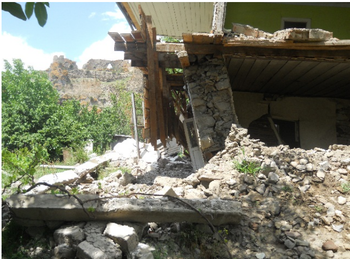
Figure 16. Village Gaghma-Atskuri landslide, destroyed house.
